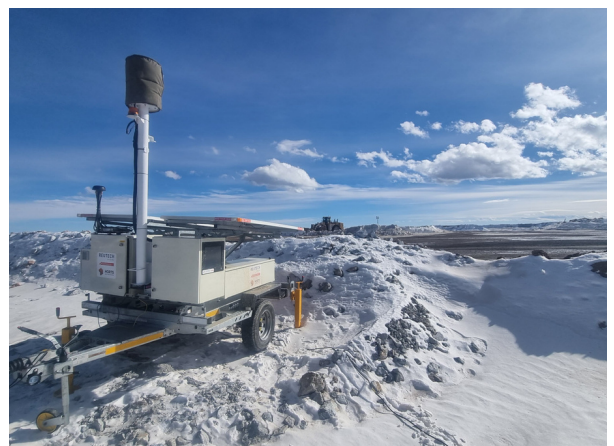
BMS deployed at -10°C
